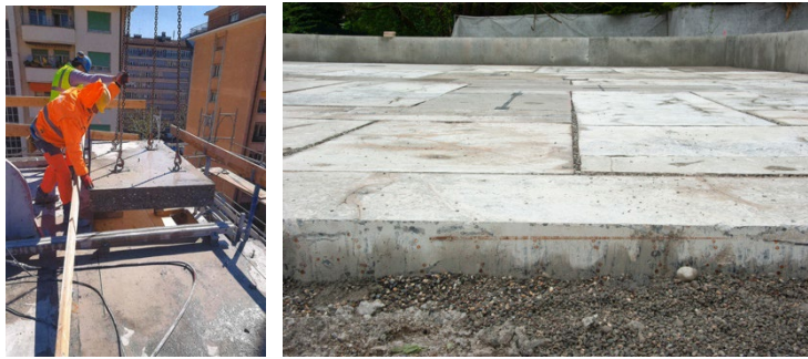
Figure 6. Concrete sourcing and reuse for the pavement of the ground floor of a building in Geneva (Ingeni SA, C. Küpfer)
